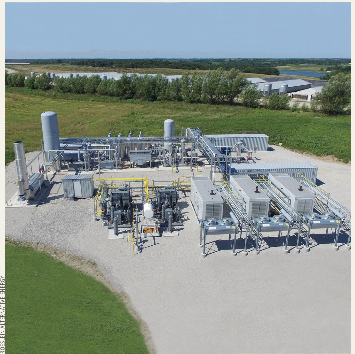
Construction is now complete on numerous farms in northern Missouri, and renewable natural gas production is underway.
